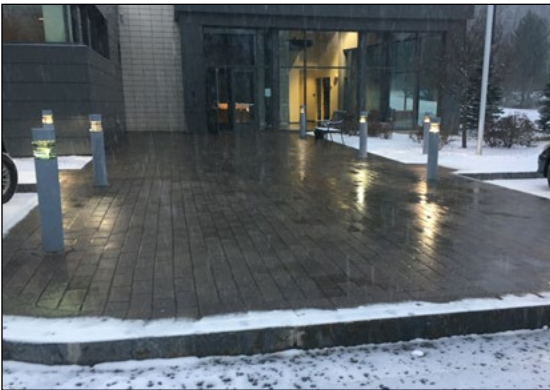
Figure B.4 Snow and Ice Melting in Operation at a Commercial Building
