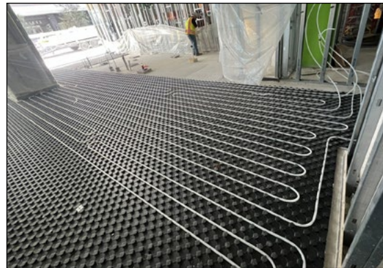
Figure B.2 Radiant Floor Heating tubing in a Commercial Application
